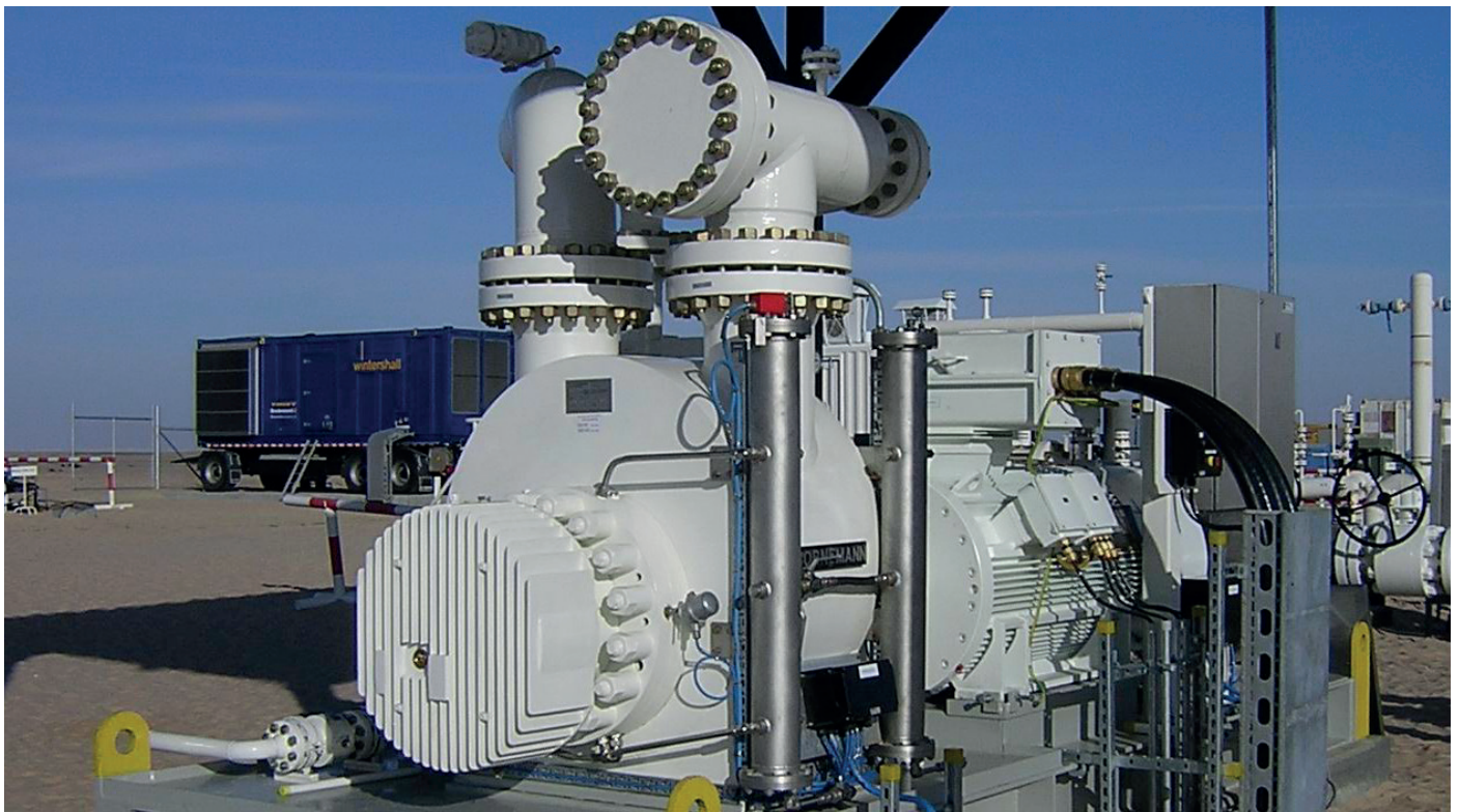
Multiphase „Boosting in Libya“
